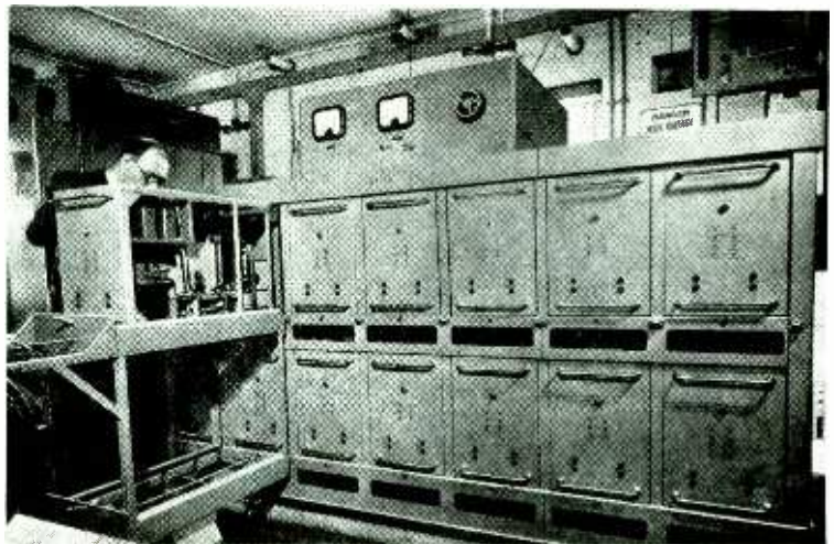
A section of the Wayne Kerr multiple-unit transmitter is shown withdrawn from its housing on the trolley provided for maintenance.
